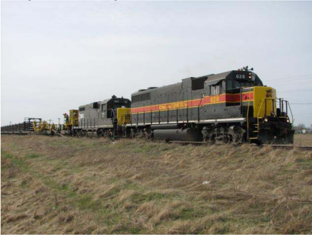
Below photos: IAIS train begins to unload the first sections of rail ribbon.
