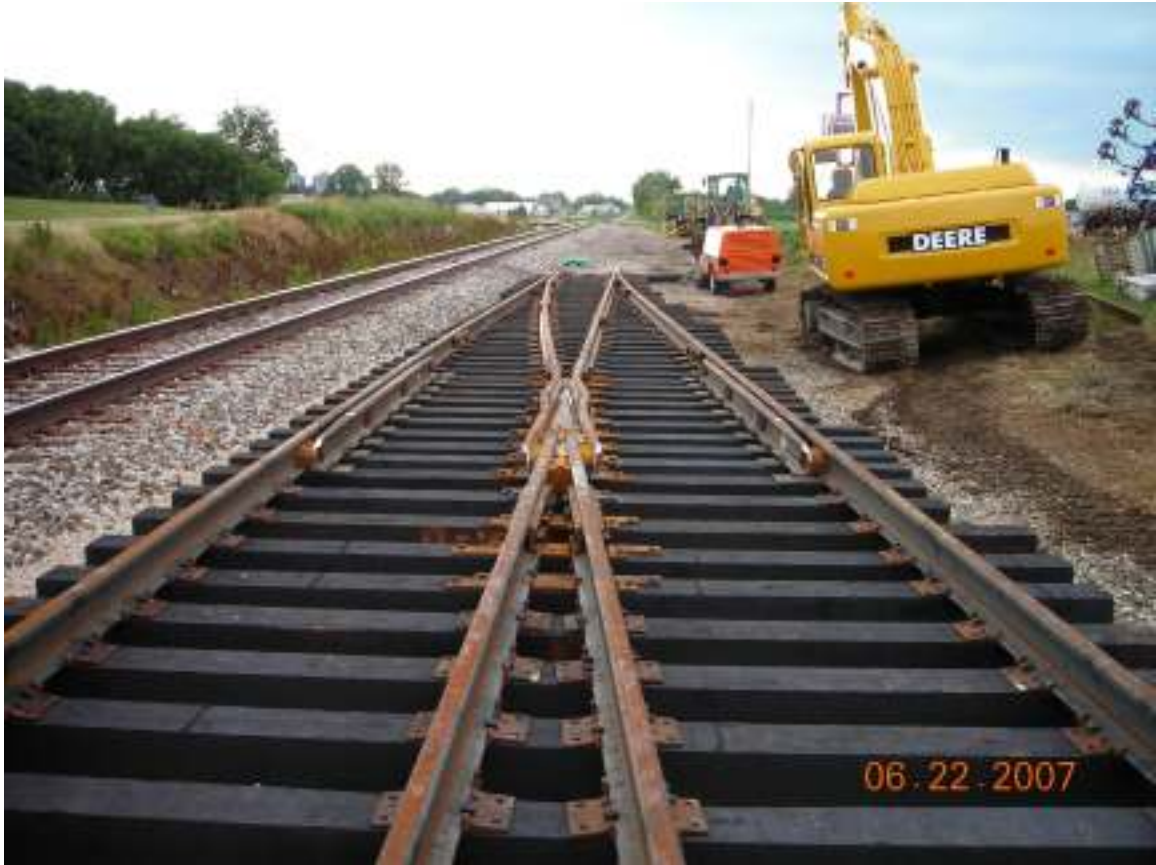
Below: First switch built at west end of siding near Annawan Co-op.
